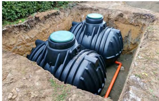
An example of a rainwater harvesting tank
